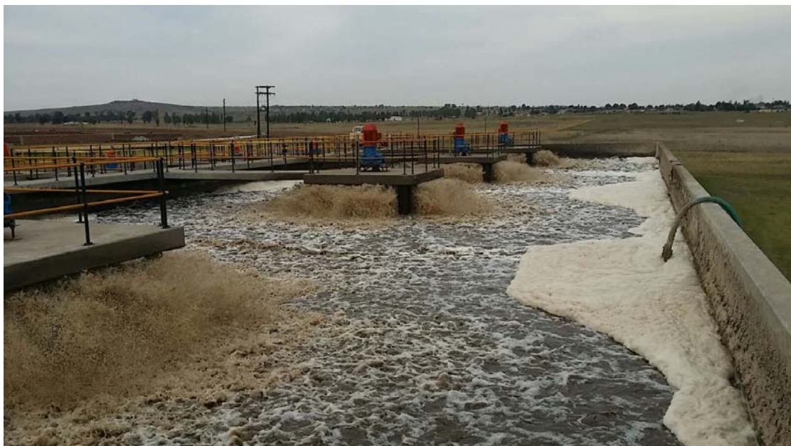
The refurbished Balfour Waste Water Treatment Works in action
